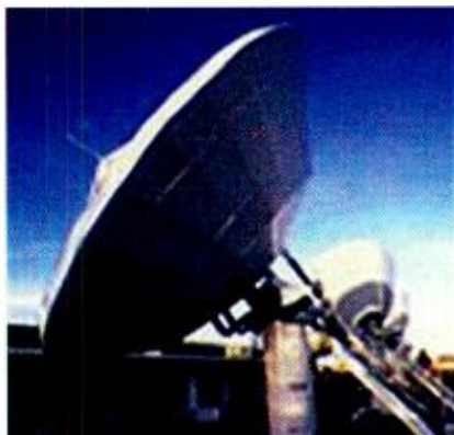
At the NDTc in suburban Denver, TCI's control room and satellite facilities will be operational, even if the power fails on New Year's Day. Officials plan to play it safe by having enough fuel on hand for emergency generators.
